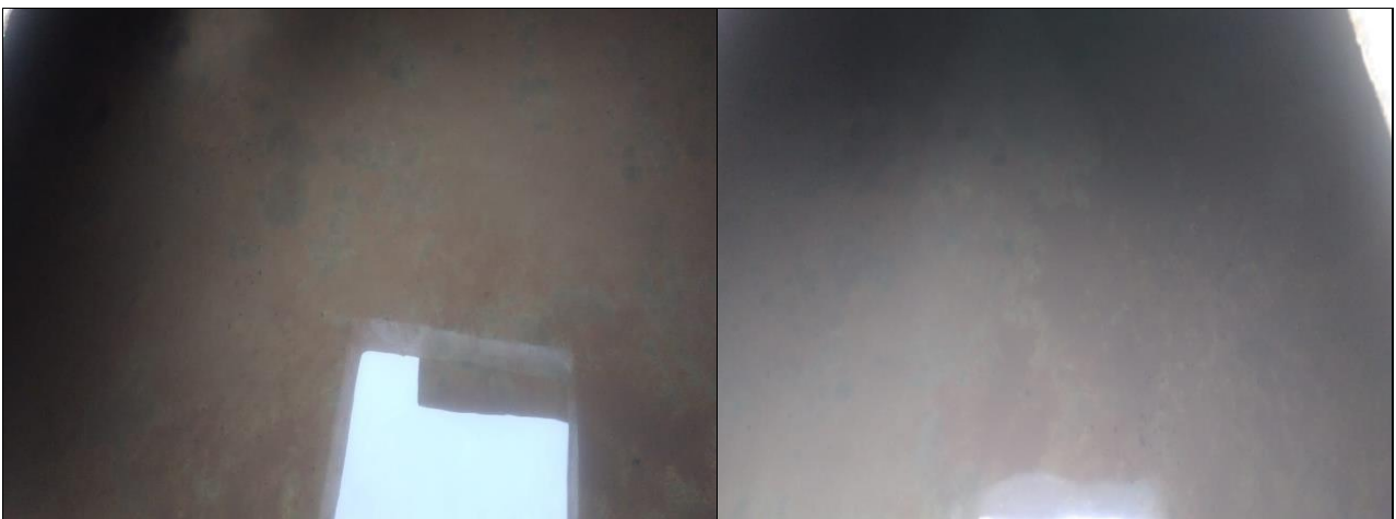
Water tank showing accumulation of silt
