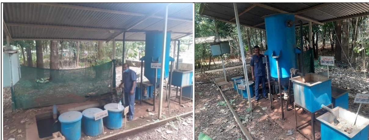
The effluent treatment plant in the Botanical Garden.
